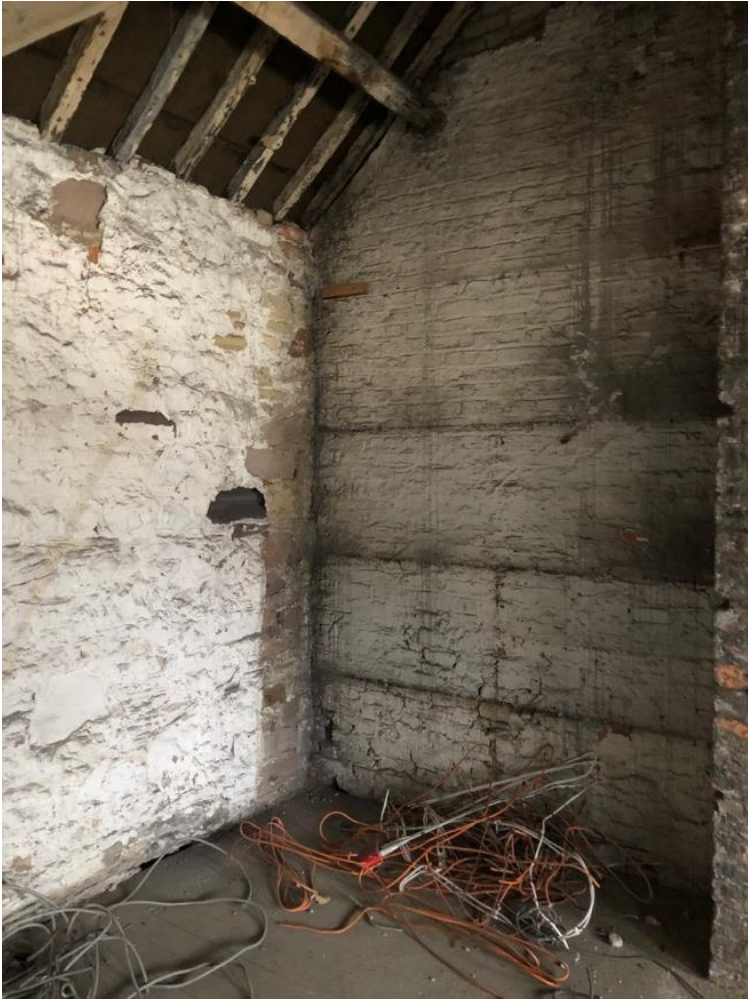
Image 18 - View of roof space to rear Party Wall showing white washed walls prior to the installation of modern dry lining. Roof in areas has been re-felted with traditional 1F felt
