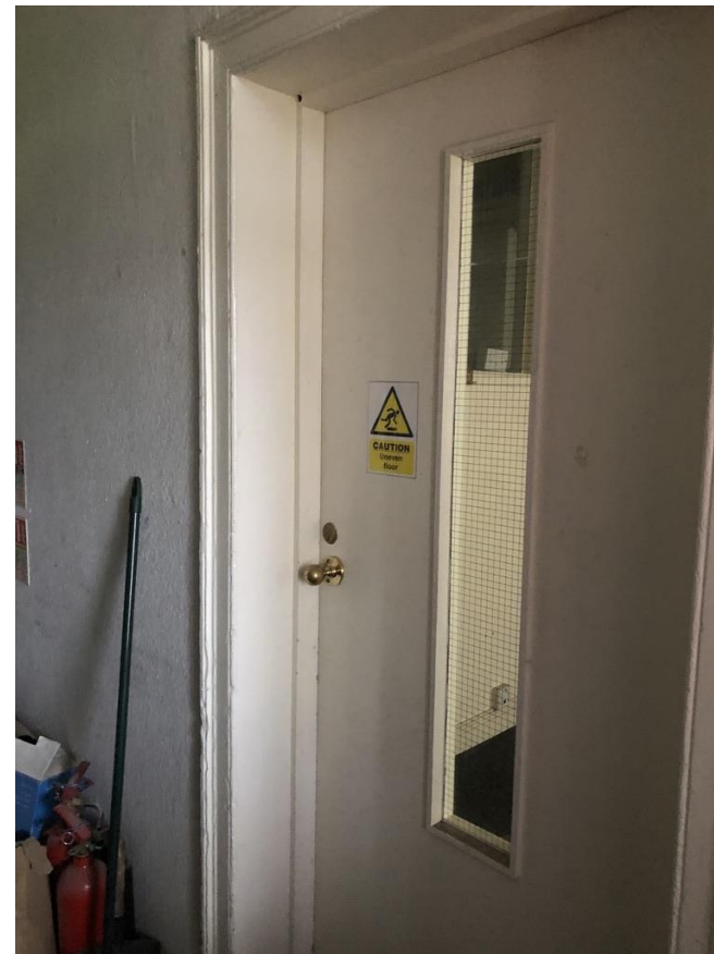
Image 10 - Front entrance door to Apartment 1 – original door lining and architraves through solid wall. Door installed is modern Fire door and wired fire glass. The proposal is to remove this door lining and architrave and make good to the plaster work. The condition of the lintol over (assumed timber) will be assessed when the works are opened up
