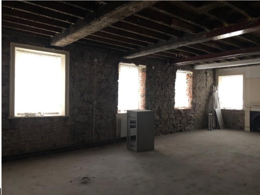
Image 14 – Reverse view of Image 11 across the first floor room. Original timber beams have been strengthened with steel work by previous owner
