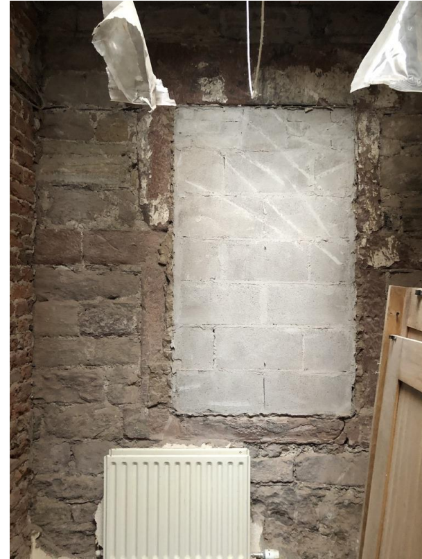
Image 6 - Existing window uncovered in original wall to rear of property, this is the location of the new doorway connecting the bedroom to the hallway in Apartment 2
