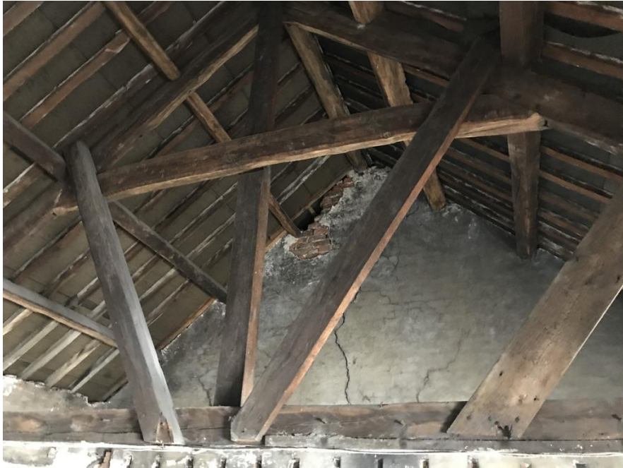
Image 20 - View to attic through existing trusses. Note additional steel strengthening added to trusses and rafter legs installed by previous owner
