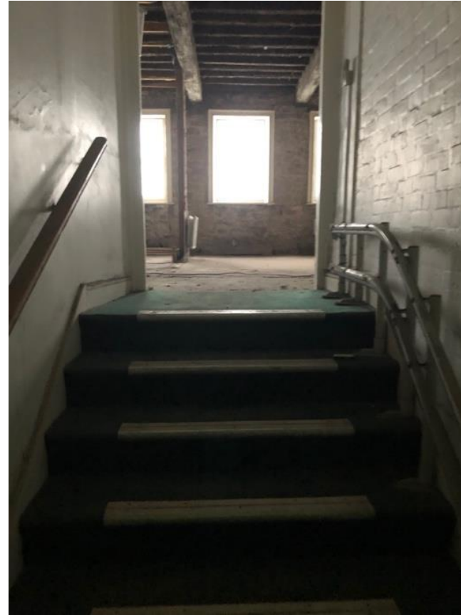
Image 23 - View from existing second floor landing with views directly through the building to the front elevation. Modern stair lift frame work fitted to right hand side of stair to be removed. No finish to existing stairwell walls currently painted brickwork
