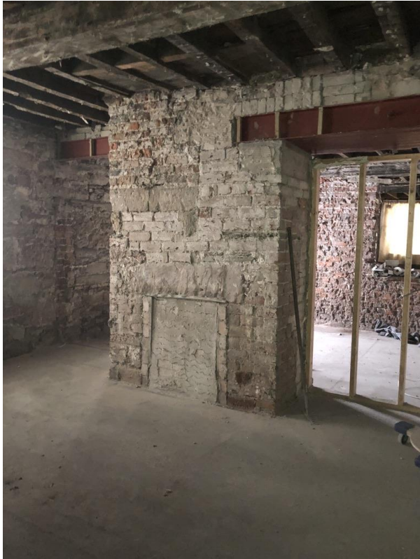
Image 5 - Internal view showing location of fireplace within Apartment 1. An existing sandstone lintol exists in this location, the fireplace has previously been removed. The openings have been strengthened with new steel beams. The window visible to the rear is the serving hatch in the former kitchen looking into the original coaching archway.
