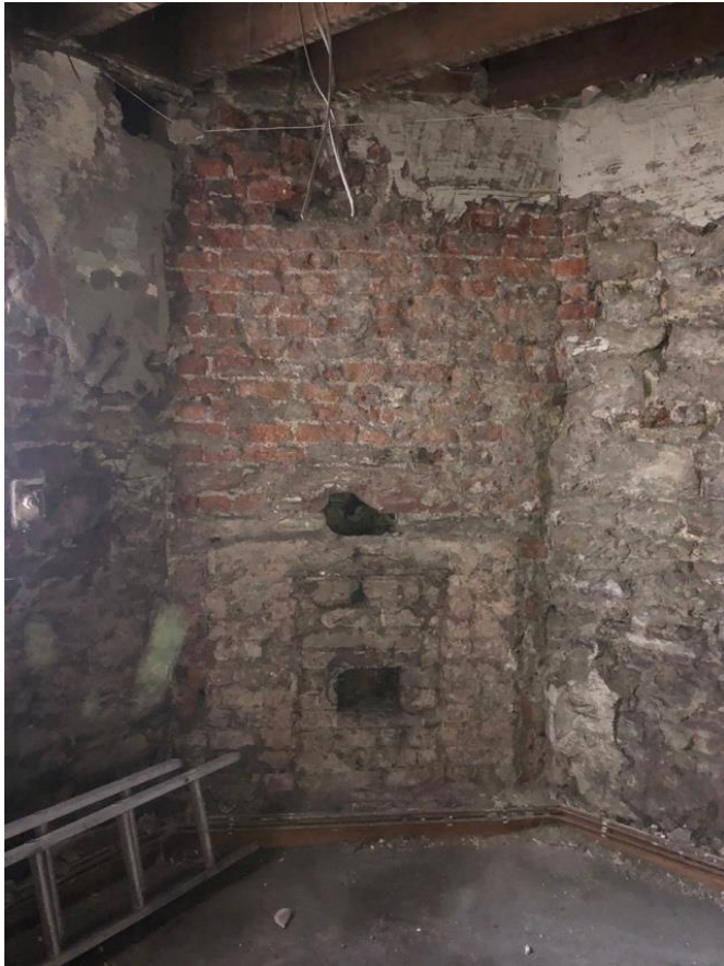
Image 3 - Proposed Cafe area – 45 degree fireplace in corner of room. Mixture of brick and stone, existing fireplace / surround has been removed. Chimney flue not visible in room above at first floor level, location of flue route to chimney stack not identified. Small pocket of similar bricks in gable wall at FF above suggesting flue may be within wall cavity.
