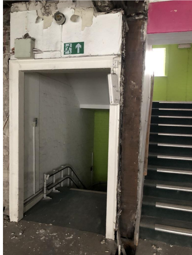
Image 17 – First floor view of staircase, right hand staircase rising to second floor. New staircase lobby re-instated to allow for continuity of 'protected stairwell' to the entrance door.
