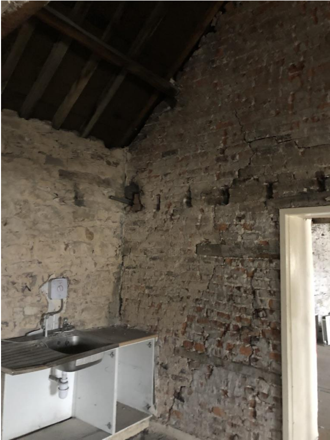
Image 22 - View of existing kitchenette to second floor, joist pockets indicate position of original timber ceiling joists – these had been removed by previous owner to install suspended ceiling throughout second floor.
