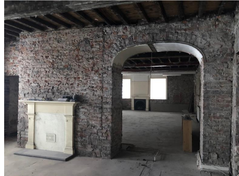
Image 15 - Original arched former on first floor dividing rooms. Note the location of the modern plasterboard stud wall approx 800mm across opening. Previously subdivision created unnatural room division. The new proposal sees inclusion of the whole arch form within the apartment and will be visible within the dressing area of Apartment 4.
