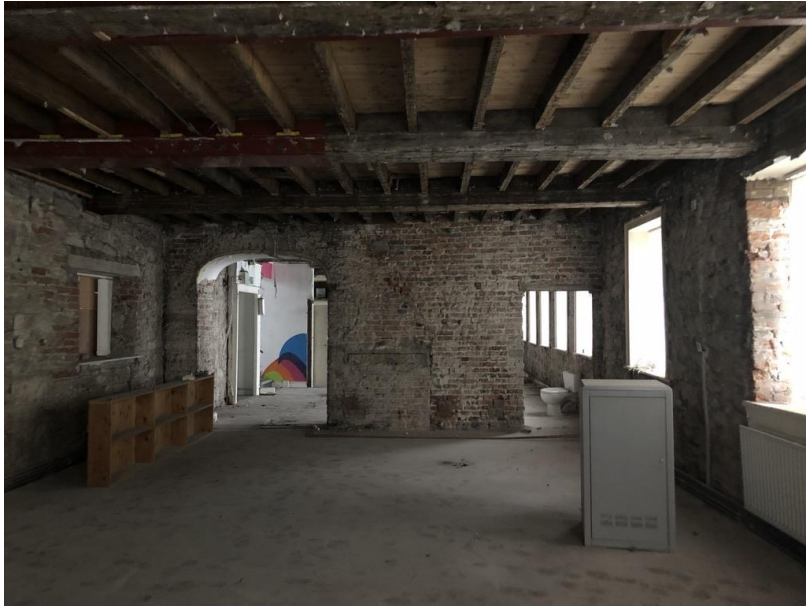
Image 11 - Apartment 3 view across open plan room, installation of bedroom wall to be fitted between the two external windows to frontage . Evidence of former fireplace in central chimney stack – existing timber infill panel to righthand side of door hidden behind plasterboard – Archway to be infilled and finished flush within the apartment. Window to left hand side to be opened up to form window to new bathroom
