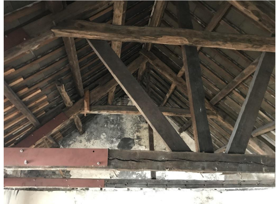
Image 21 – Additional steel strengthening added to trusses and rafter legs installed by previous owner – part replacement roof rafters to rear pitch of roof. The proposal is to insert a mezzanine floor level within this roof zone to provide a bathroom and study to Apartment 5. The works will not require any alteration to the trusses and allow them to be exposed within the finished building rather than hidden behind suspended ceilings. The new staircases are designed to fitted between trusses. New rooflights are fitted between the existing purlin positions
