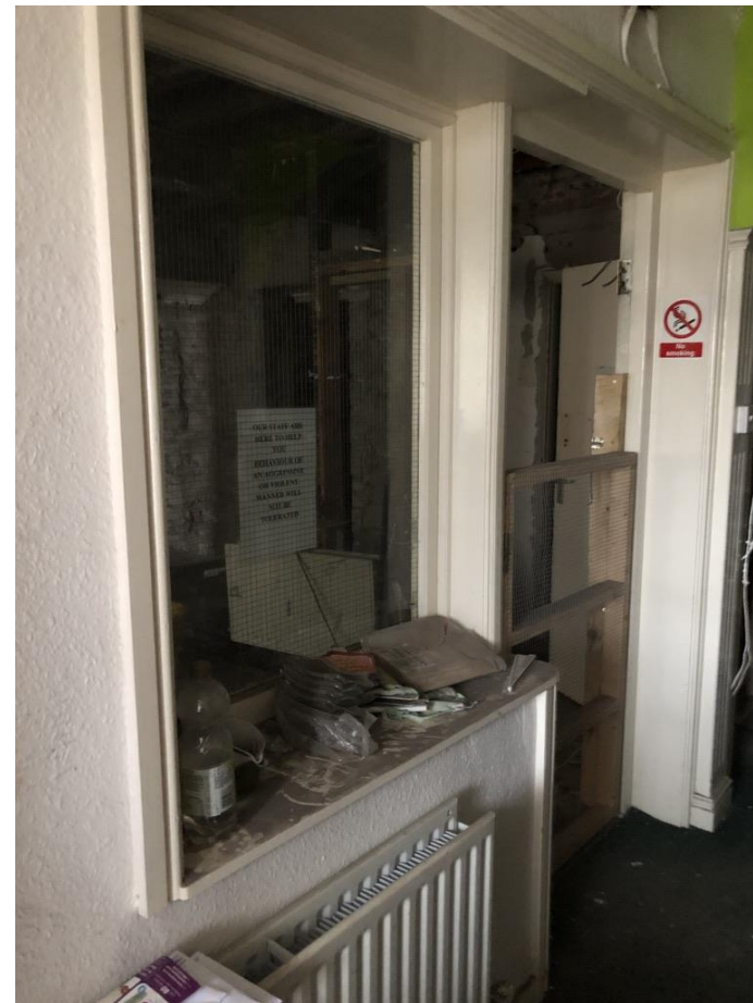
Image 2 - Ground Floor entrance screen into Apartment 1. Screen formed in softwood Torus profile with wired fire glass to provide fire integrity to wall. Screen and door made in modern planed timber. Proposal is to remove the screen and re-instate the wall in new masonry to the full width of the wall, the existing lintol will be retained in-situ to avoid further disturbance to the structure.
