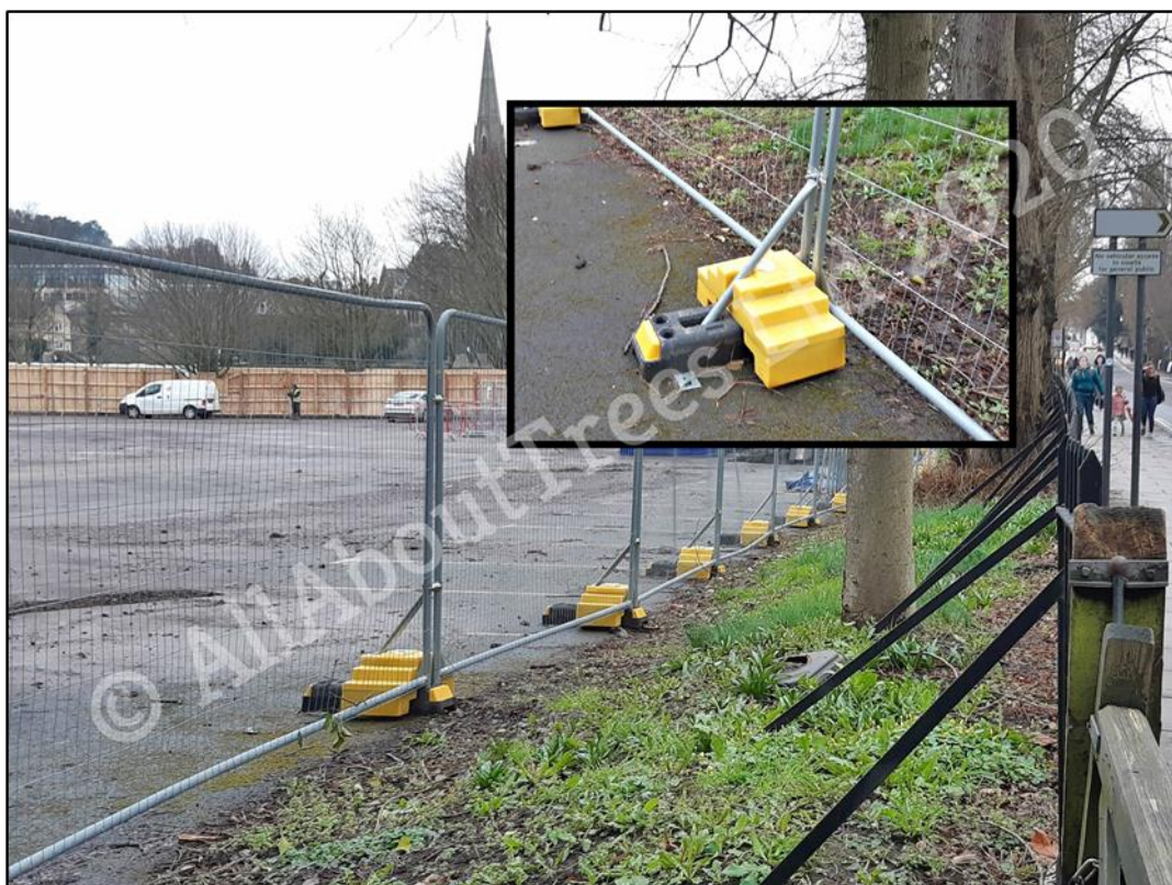
Figure 4 – An example of a barrier erected on a site
