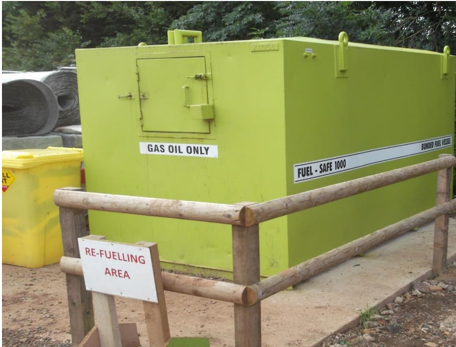
Figure 9 - Example of a protected refuelling area on handstand with spill kit
