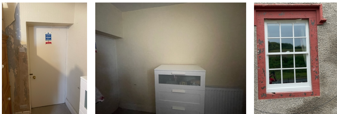
Images 10, 11 & 12: bedroom door/opening to be retained, wall where proposed opening is to be formed & new double glazed timber sliding sash as installed in the main house as part of recent approval.
