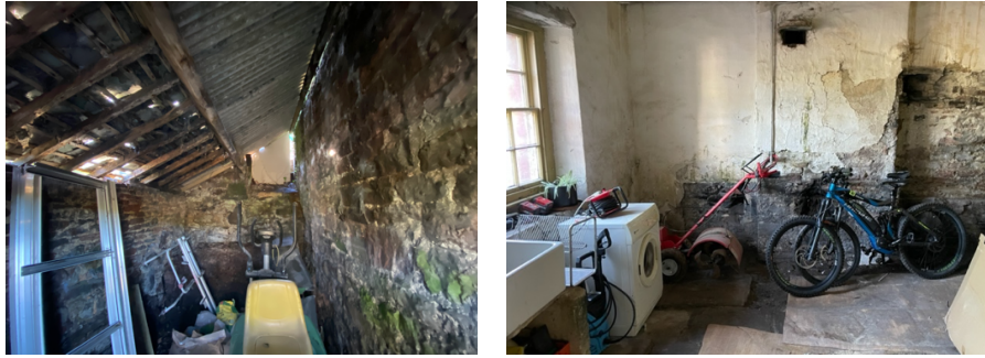
Images 12&13: External store roofline raised & Openings formed both sides of chimney breast.
