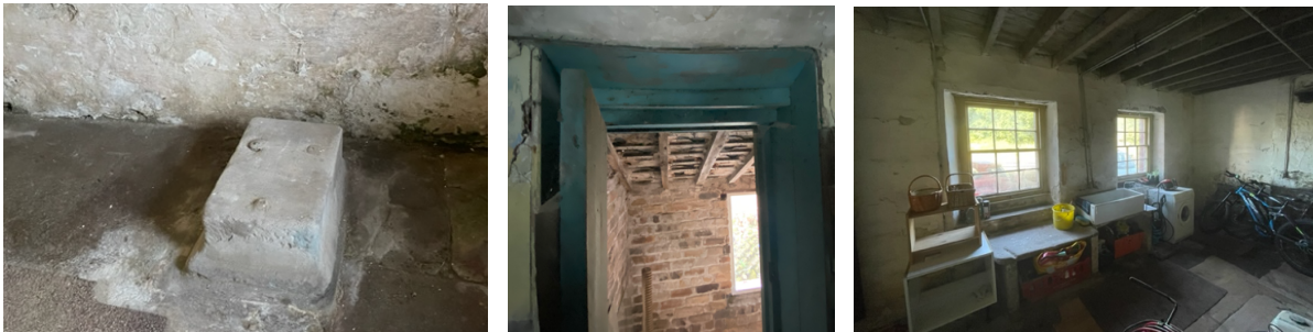
Images 7,8 & 9: Stone plinth with concrete bedding, Lining to first floor door opening & GF Utility
