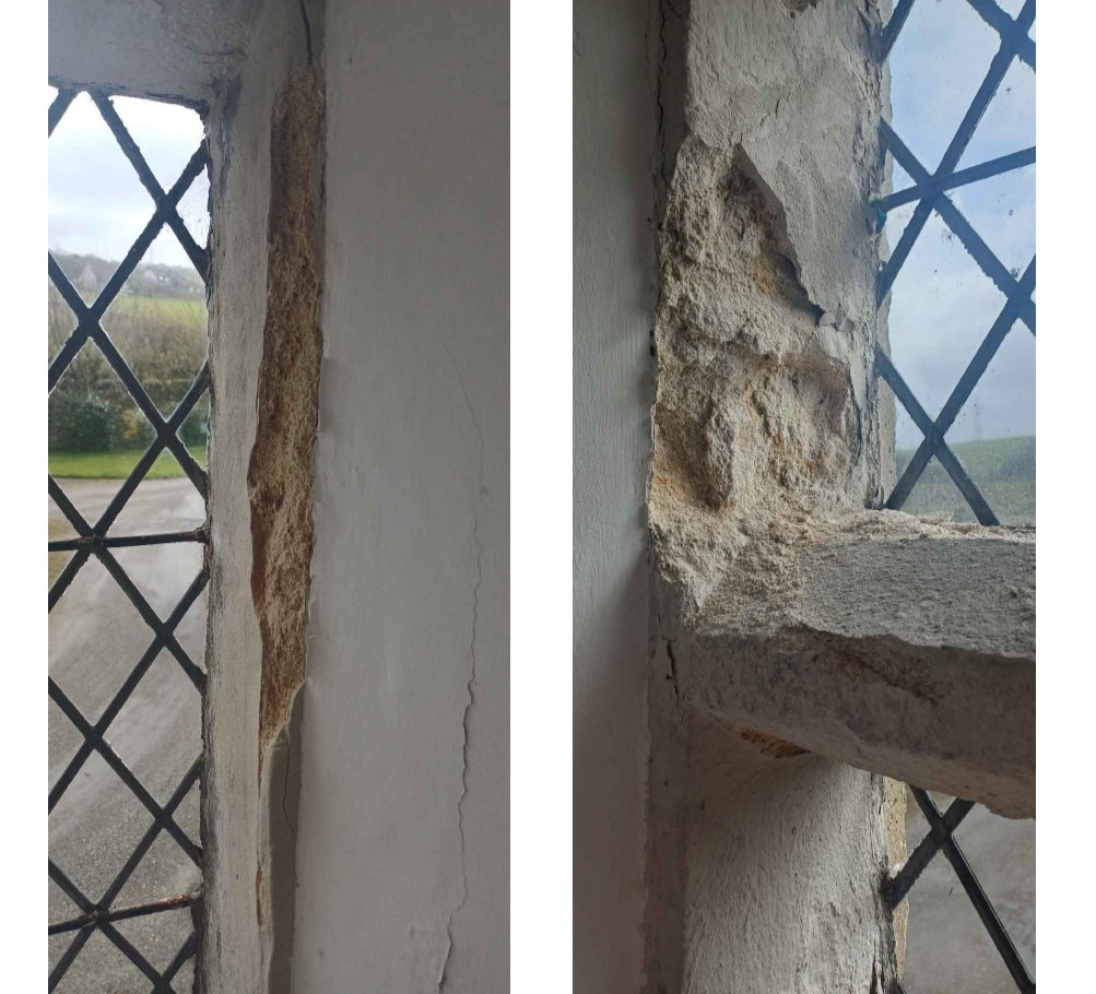
Photographs of typical internal stonework deterioration to existing windows.
