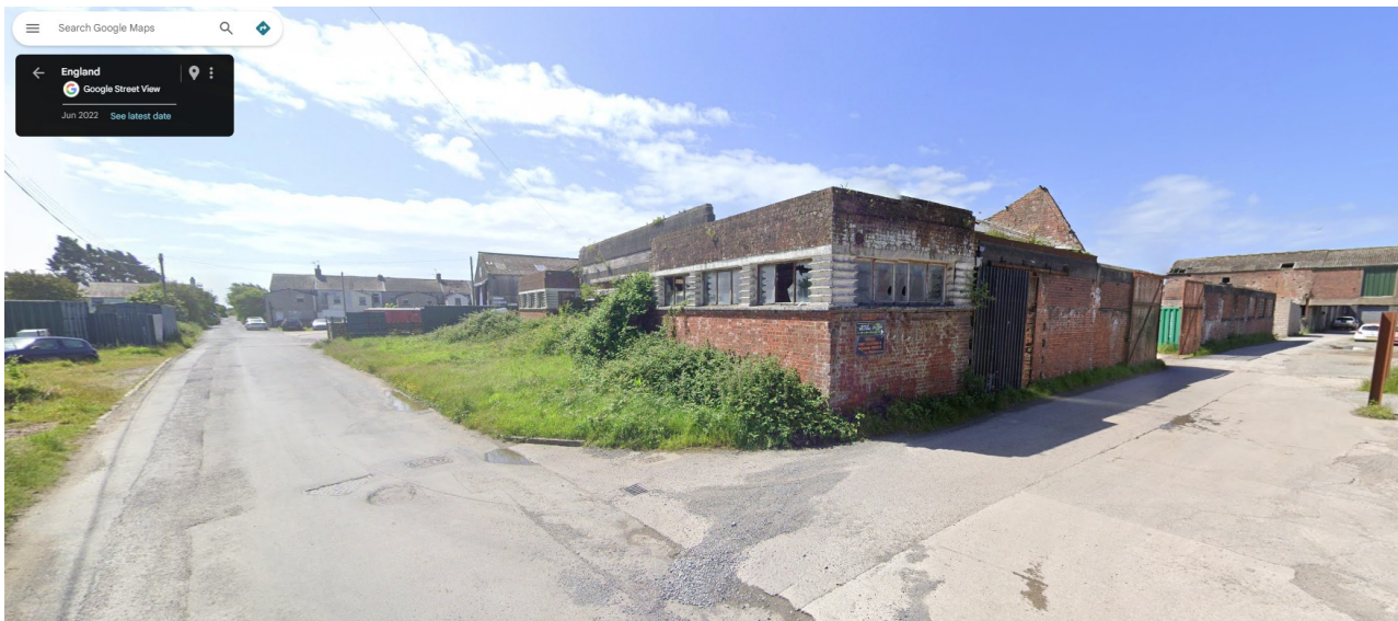
4 The Tannery as existing in 2022. Efflorescence is visible on the entirety of the building. Vegetation has encroached the entire façade and most windows have been broken, allowing the elements to deteriorate the inside of the building.
