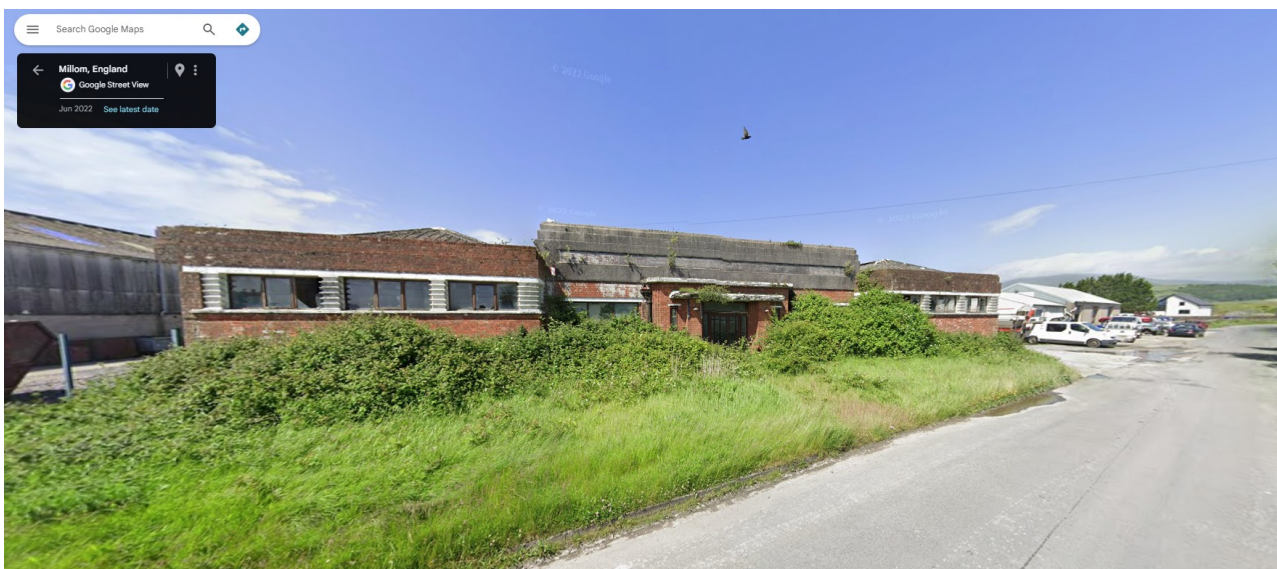
5 The Tannery as existing in 2022. Vegetation has encroached the entire frontal elevation and can be seen establishing itself on the decorative concrete elements above the main entrance.
