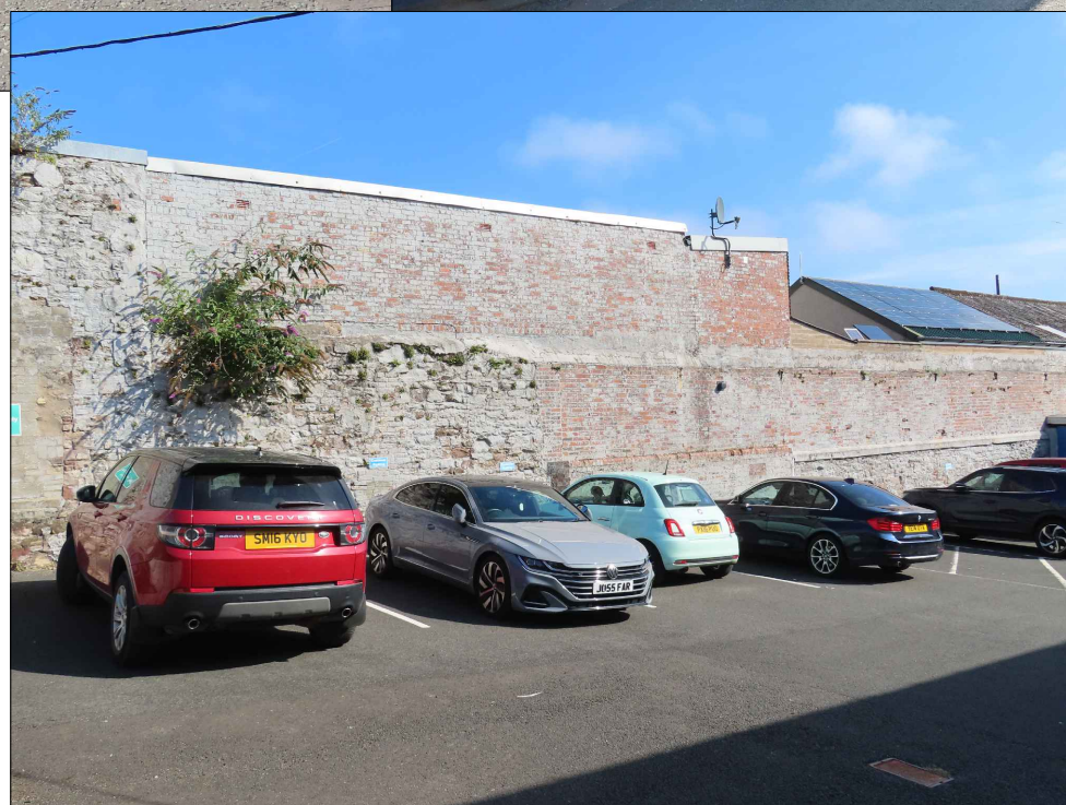
This picture shows the rear of the building. 75% is pointed brickwork there is a small section of un-rendered masonry but the application works do not include any alteration or extension to this elevation.
