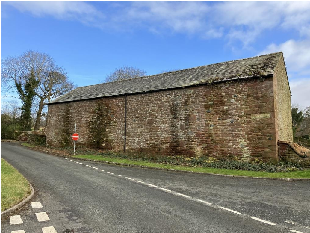
Roadside barn elevation – two rooflights inserted in slope to retain overall visual amenity of the barn
