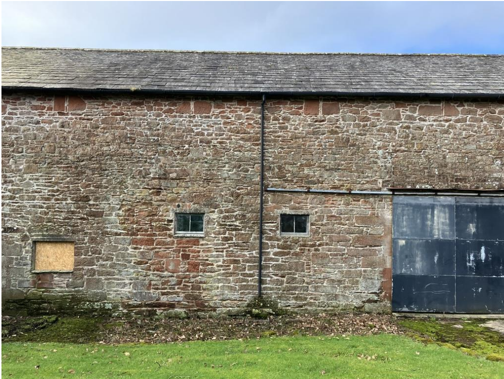
Existing windows to be enlarged to suit the new use with sandstone quoins and lintols
