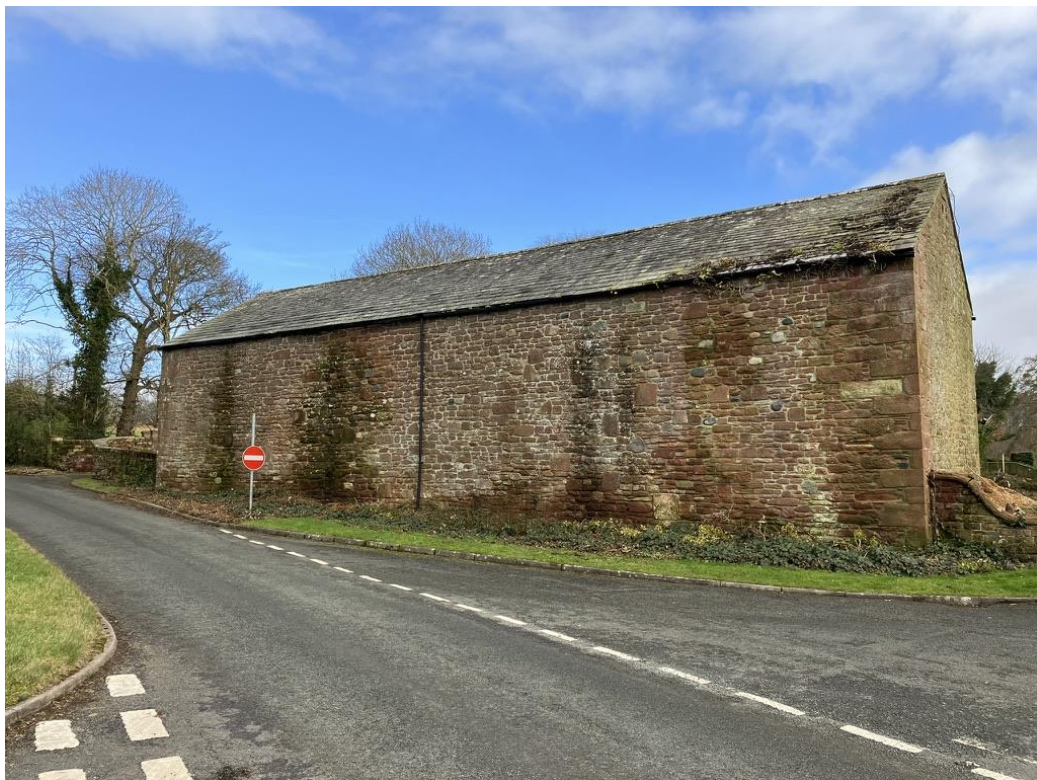
Roadside barn elevation – five rooflights inserted in slope to retain overall visual amenity of the barn
