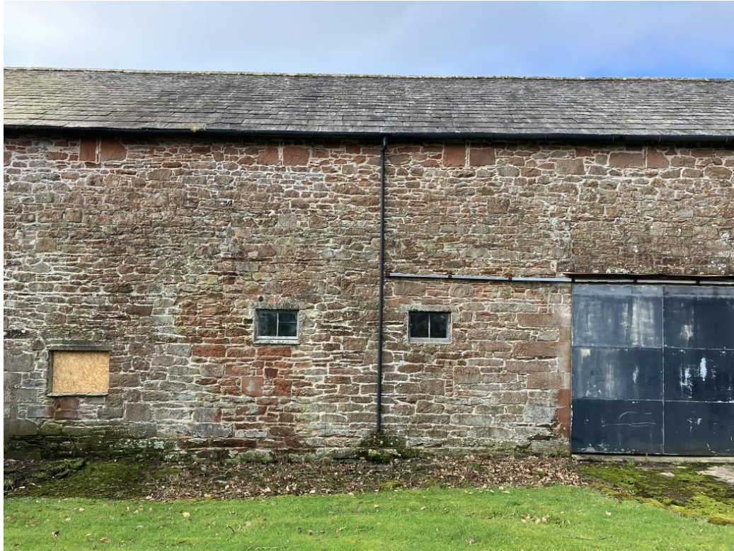
Existing windows to be enlarged to suit the new use with sandstone quoins and lintols
