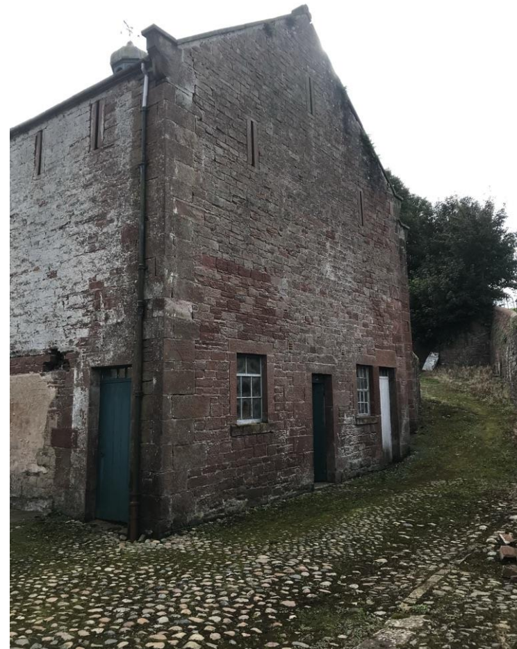
North Gable elevation with retained cobbled paving, upper floor new windows designed to reflect detailing of the lower ground floor windows
