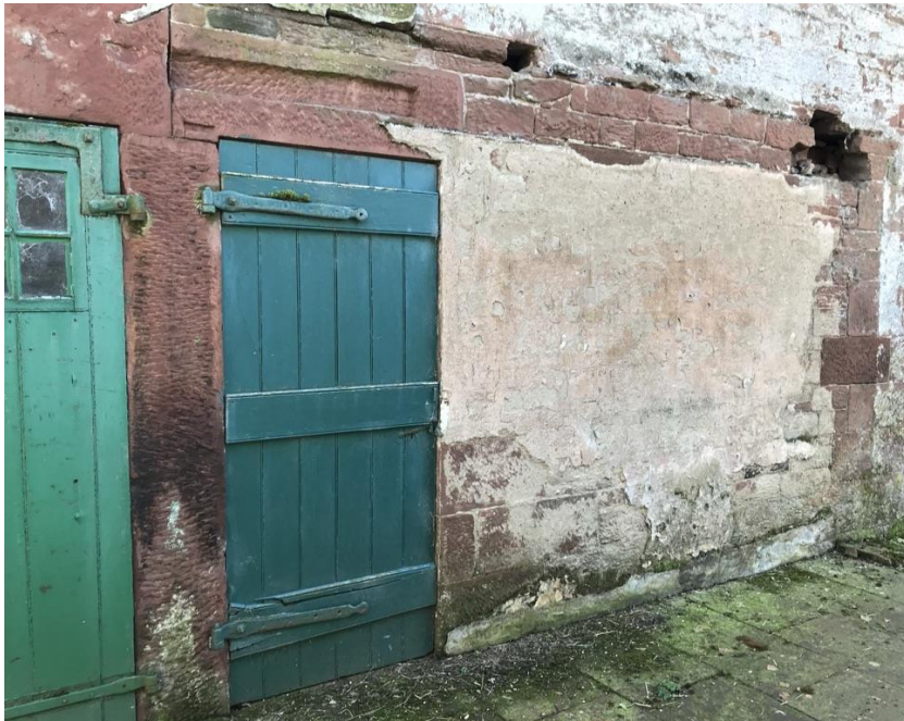
Limewash to existing wall in area of previous structure. Stonework to be patched into existing wall and sourced from sandstone on site
