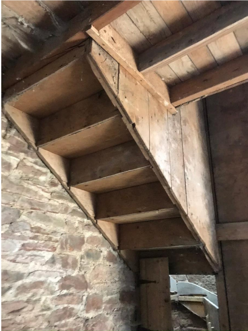
Access stair to pigeon loft - collapsed winder stair shown preventing access to loft level
