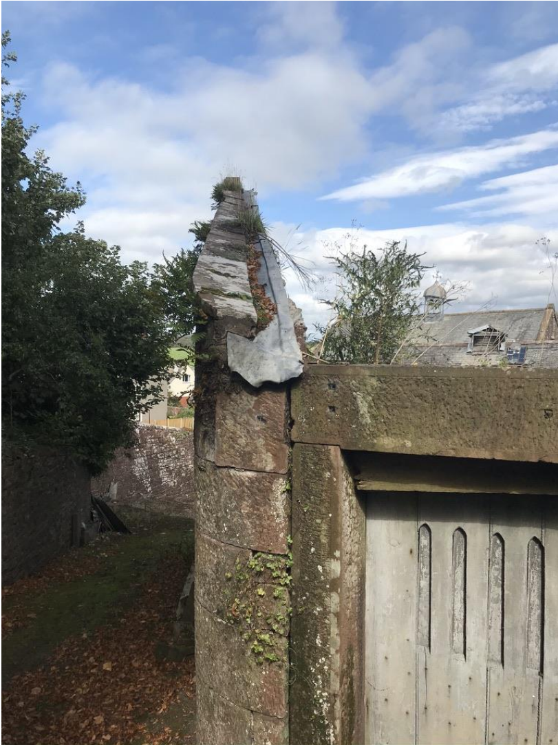
Remaining elements of the stable / boiler house with parapet and leadwork in tact, roof has been collapsed for over twenty years. Works will stabilise the wall and allow long term retention of the built form.
