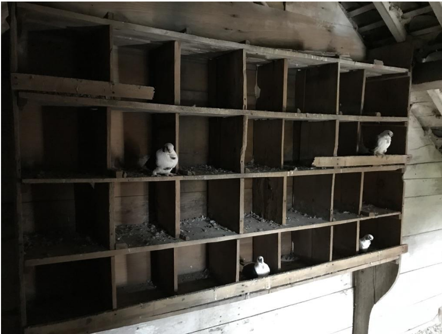
Original photo 2019 prior to access stair becoming unsafe
