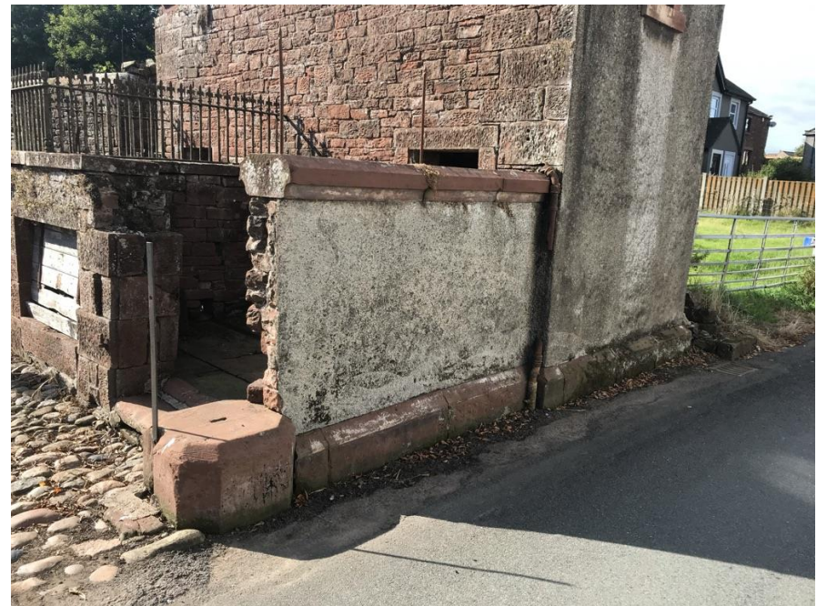
Former gate stoop to North corner of site - matching gate stoop to South corner of gate now lost as part of earlier entrance widening
