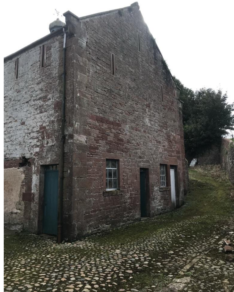
North Gable elevation with retained cobbled paving, upper floor new windows designed to reflect detailing of the lower ground floor windows
