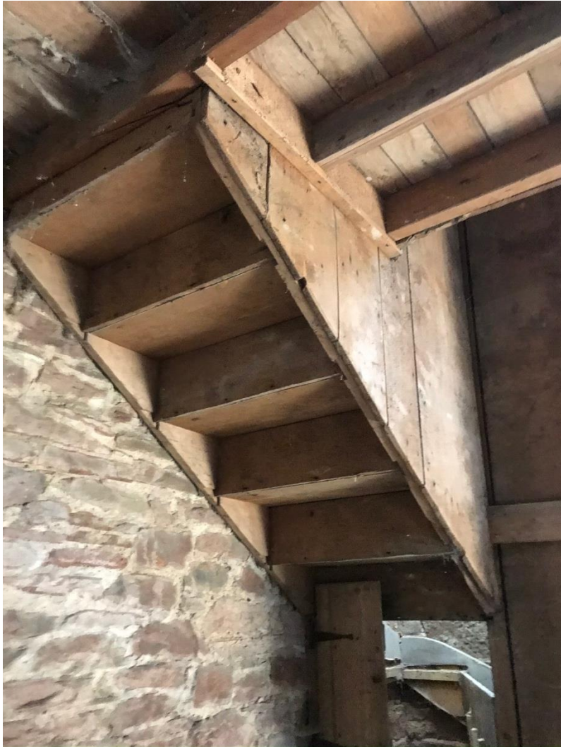
Access stair to pigeon loft - collapsed winder stair shown preventing access to loft level
