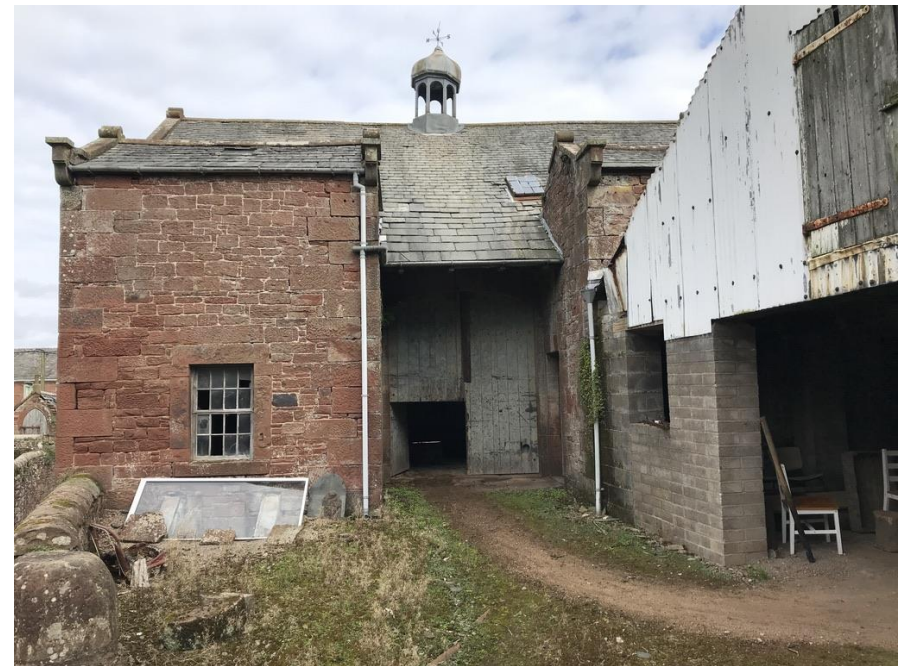
View looking East, modern gin house wall to be moved back to allow view of existing symmetrical turreted sandstone rear outriggers
