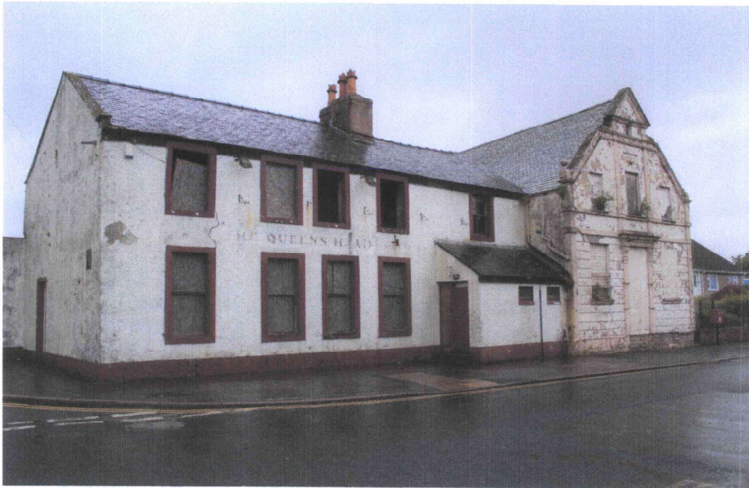
View of former Pub & Chapel from the south, with house sparrow , swallow & jackdaw entries
