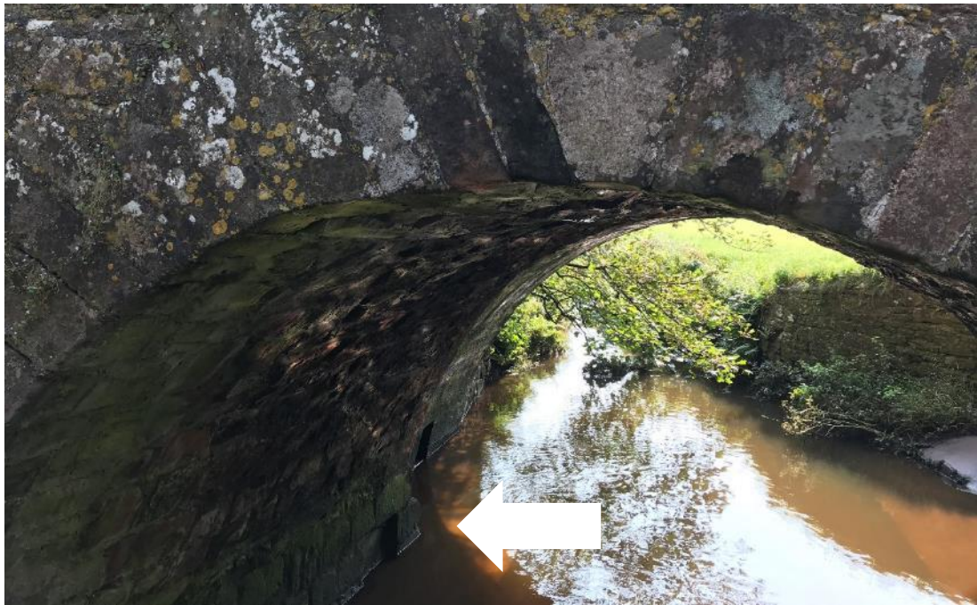
Figure 10 The grade II* listed bridge over Pow Beck, with the join between the 16 th century original arch (the nearer section) and the later part (further away) indicated. On top of the bridge, the difference can also be appreciated in the different levels of weathering of the east and west parapets.
