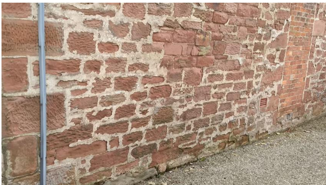
Figure 105 Poor quality pointing risks harming the characteristic appearance of St Bees' red sandstone. In certain cases, it will be contributing to damage to the fabric of the stone itself. This is particularly apparent where stone surfaces have delaminated or powdered away, leaving an edge of pointing standing proud.
