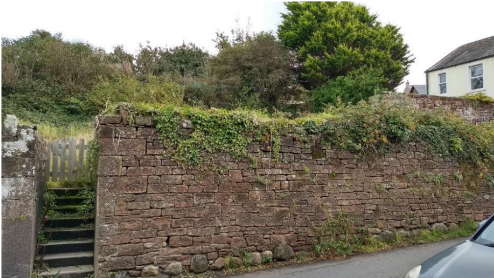
Figure 76 The attractive wall (its cock-and-hen coping stones are obscured by ivy) separating the road from an area of vegetation that, like the barn at Town Head Farm, allows the area to retain aspects of its agricultural history. Sites like this are vulnerable to infill buildings, or even pressure from car parking. The gradient of this plot has likely been its saving grace by making such development difficult.
