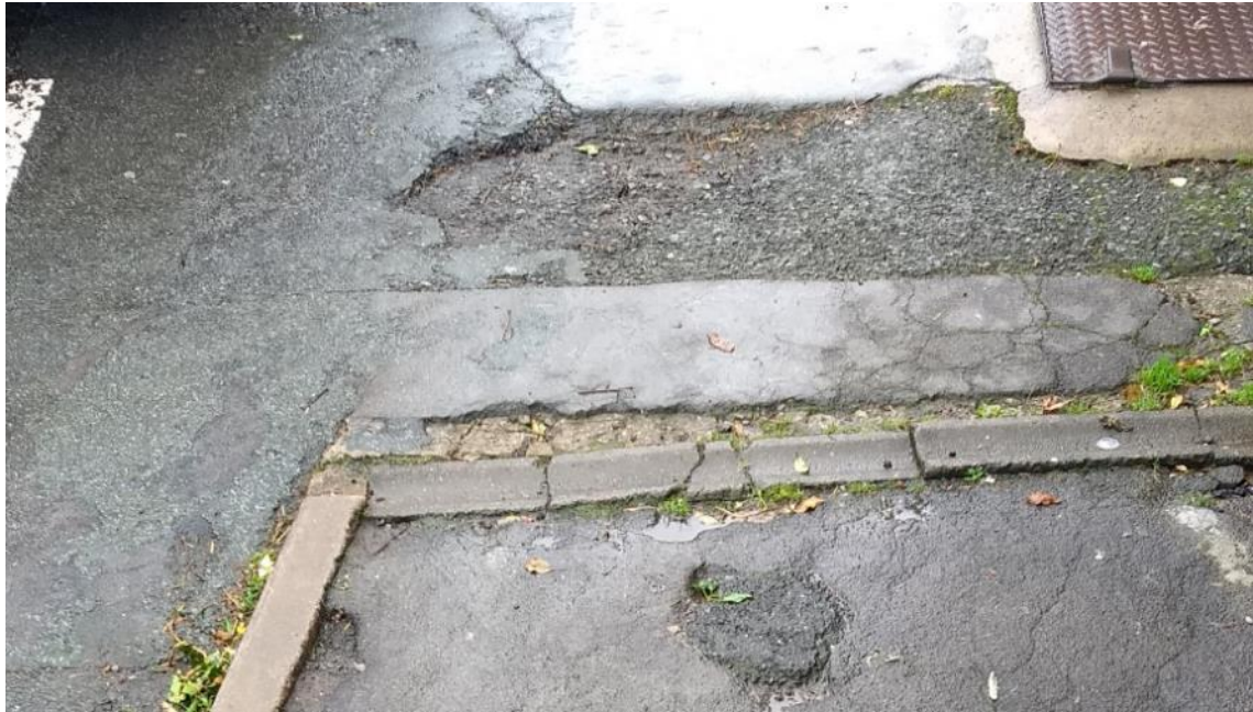
Figure 95 Tarmac causes more problems the older it gets. Any movement beneath it results in cracking, and repair leads to mismatched patches that move and wear relative to the original. Eventually, an unsightly mass of scarred material results, and furthermore contributes to surface water runoff.
