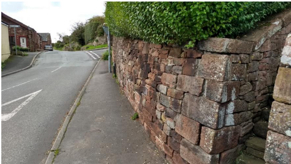
Figure 102 This wall on the corner of the B5345, just outside the boundary of the conservation area, is quite noticeably bulging. Many of the walls in this area are retaining walls, and the mix of little slopes and steps cut into the incline is characterful. However, these retaining walls need monitoring to make sure they do not lose integrity.
