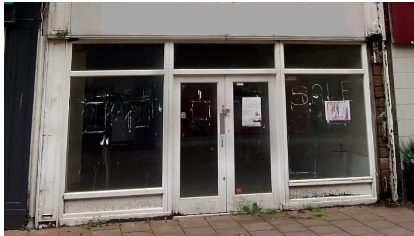
Figure 20 A shopfront where the right pilaster has been rotted away by a missing rainwater pipe that has run water over it without being fixed.
