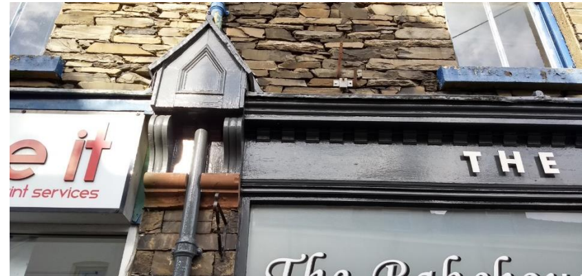
Figure 24 Here, the gablet (small gabled element) is deep enough to have its own lead capping, with the downpipe neatly integrated behind, between stone blocks that subtly resemble the curved console brackets underneath the gablet.
