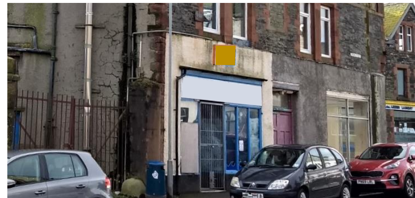
Figure 22 This shopfront's difficulties are compounded by the dilapidation of the building it's attached to.
