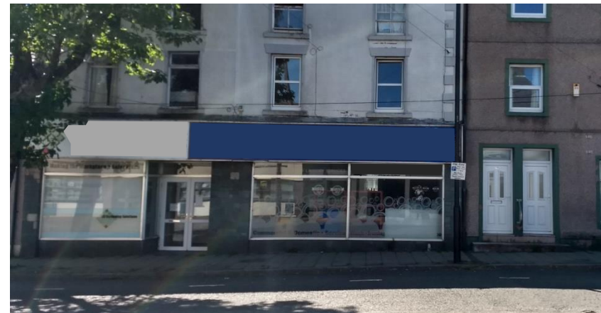
Figure 14 These shopfronts are not accordant with rules of proportion. The lack of pilasters causes vertical emphasis, and definition of bays and plot widths, to be lost.
