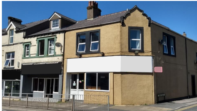
Figure 12 This shopfront has lost its original corner door, undermining the architectural effect.
