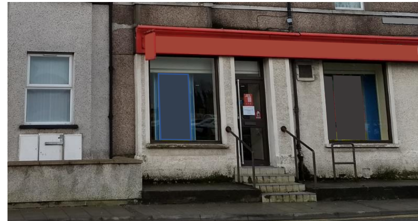
Figure 21 Algae and dirt caused by rain splashing on the base of the render. This is an easy fix with cleaning and repainting, if the render is sound.
