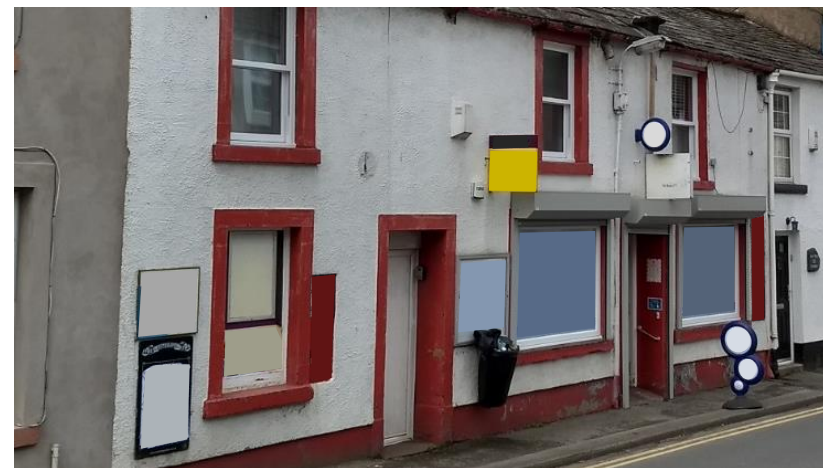
Figure 19 This building has accumulated a number of accretions over the years that prevent it looking as good as it might: signage without a consistent appearance including projecting signs, lighting, cables, a litter bin, alarm boxes, and external shutter boxes.
