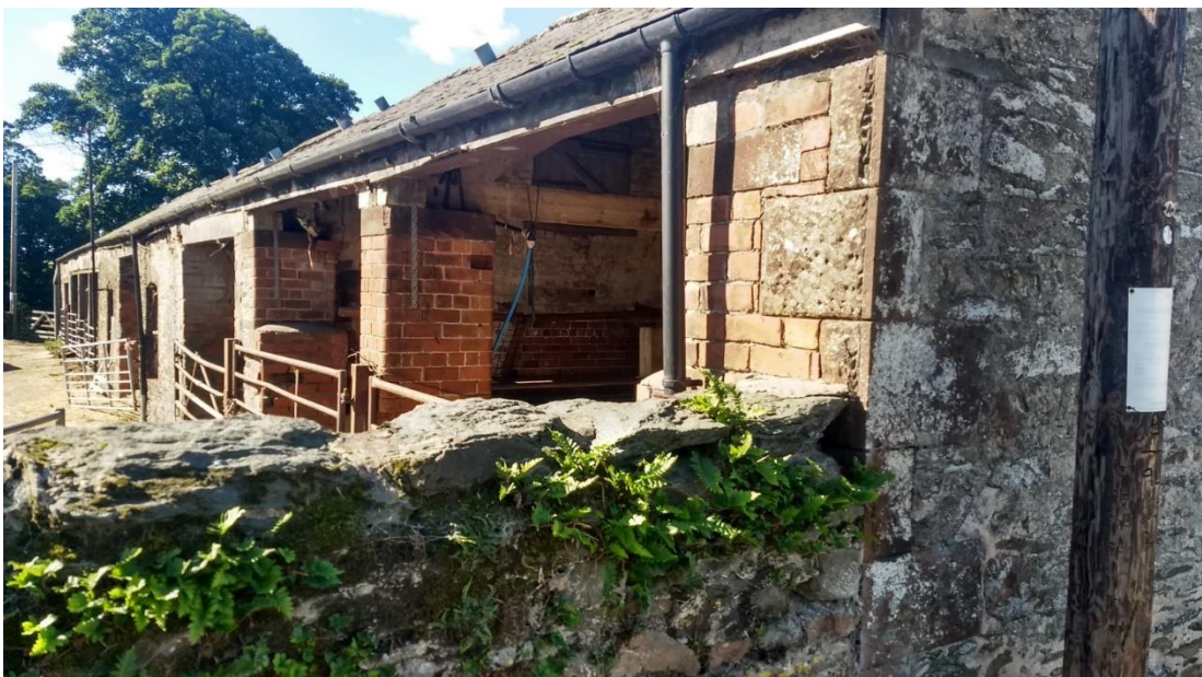
Figure 18 This old wall adjacent to the byre has small ferns growing in the top that enhance its character. Plants can, however, cause damage in masonry when left unchecked.
