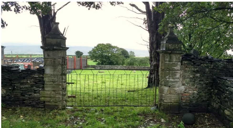
Figure 8 One of the pairs of grade II listed gate piers, to the east of the castle ruins. One of the ball finials appears to be lying nearby.
