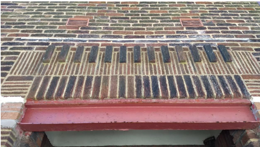
Figure 18 Sunday school doorway on Earl Street. This excellent brickwork would greatly benefit from the replacement of the RSJs with something more subtle, and greater care in future repairs with the pointing.
