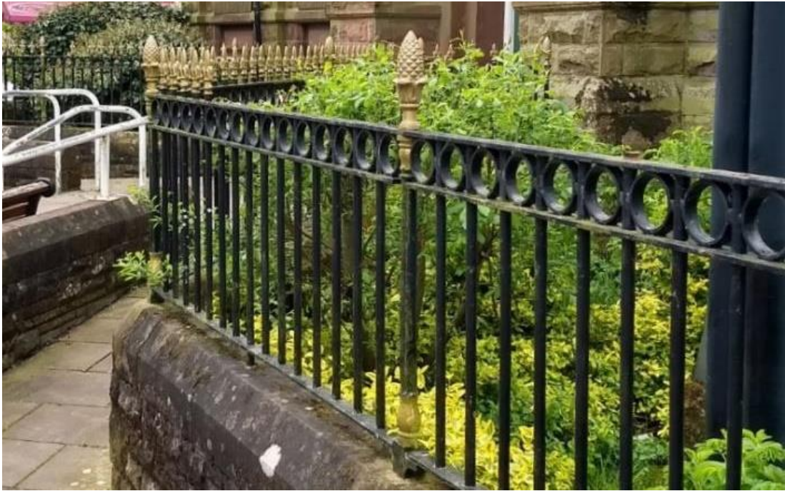
Figure 11 Iron railings, dating from the early 1990s
