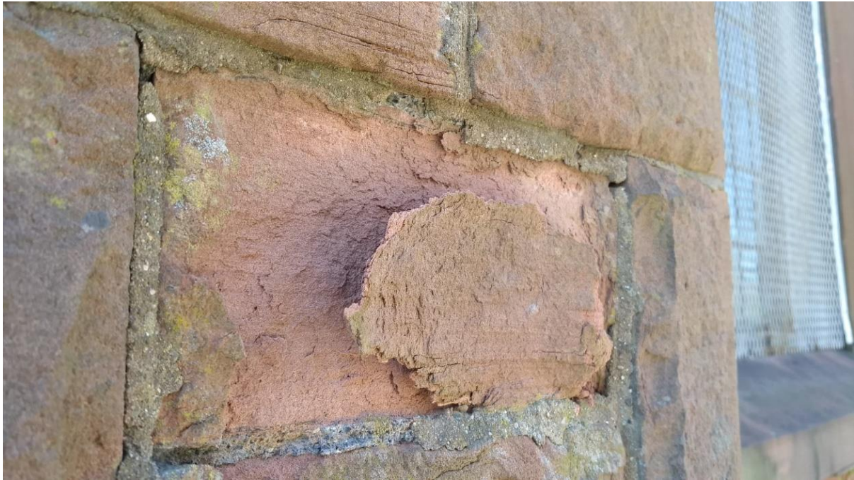
Figure 43 The side elevation of the Methodist Church bears particular witness to the damage that can be caused by hard cement pointing. Much of the stone has delaminated and powdered as a result.
