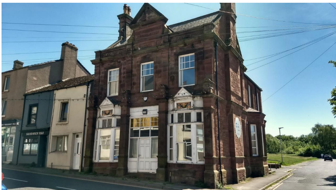
Figure 31 The former conservative club of 1883. Note the ornamentation to the windows and the lettered frieze and pediment at the top. Timberwork such as this is vulnerable and requires regular inspection.
